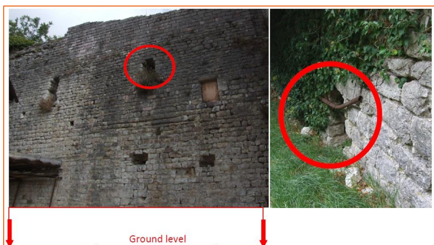
Figure 11 - zone 3-4: Walls downstream side (on the left) and upstream (on the right) - notice the opening at around 6 metres from the ground level downstream and the same opening at ground level on the right.
