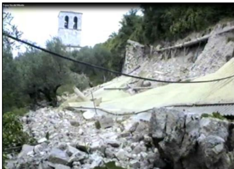
Figure 17 – ancient wall collapse in via del Monte
