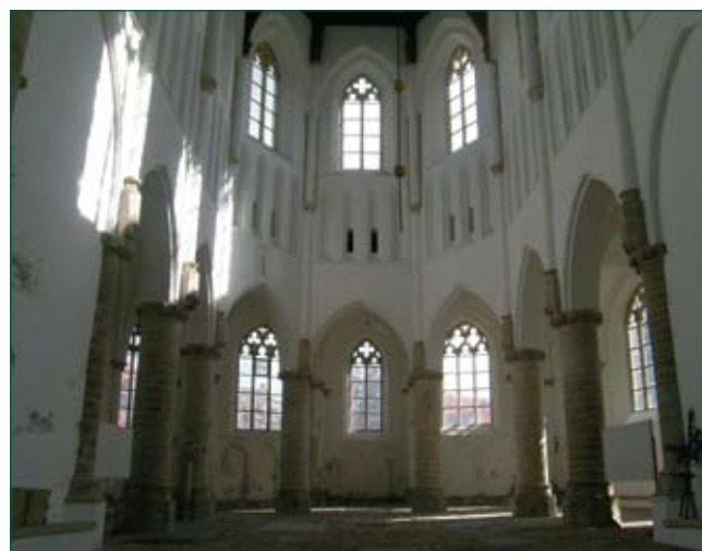
Damage to plaster due to salt, RH cycles leading to irreversible dilation
