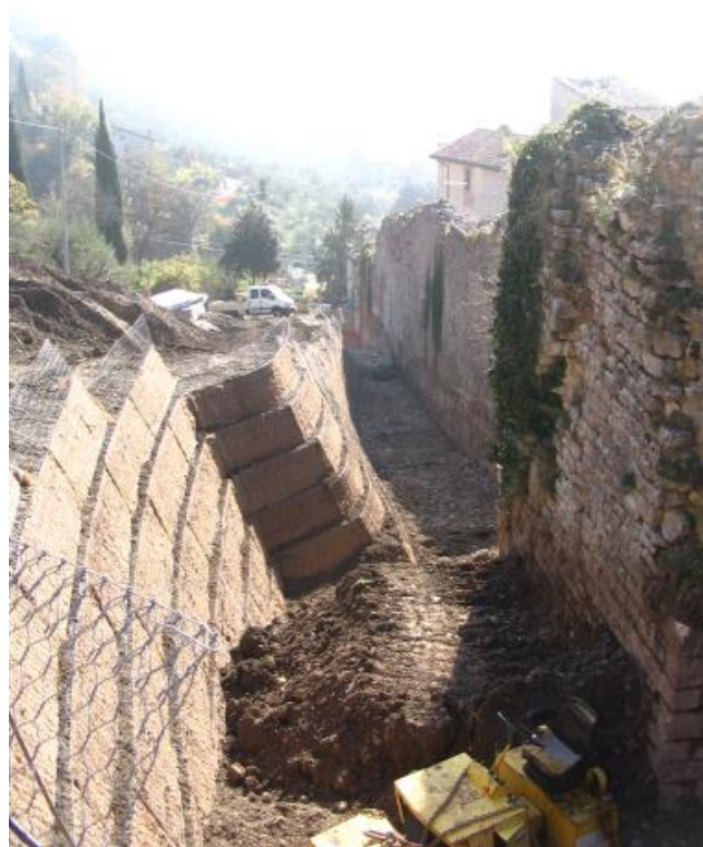
Figure 10 - town Walls: upper part - the slope AFTER intervention with a clear vision of the retaining/reinforced earth wall
