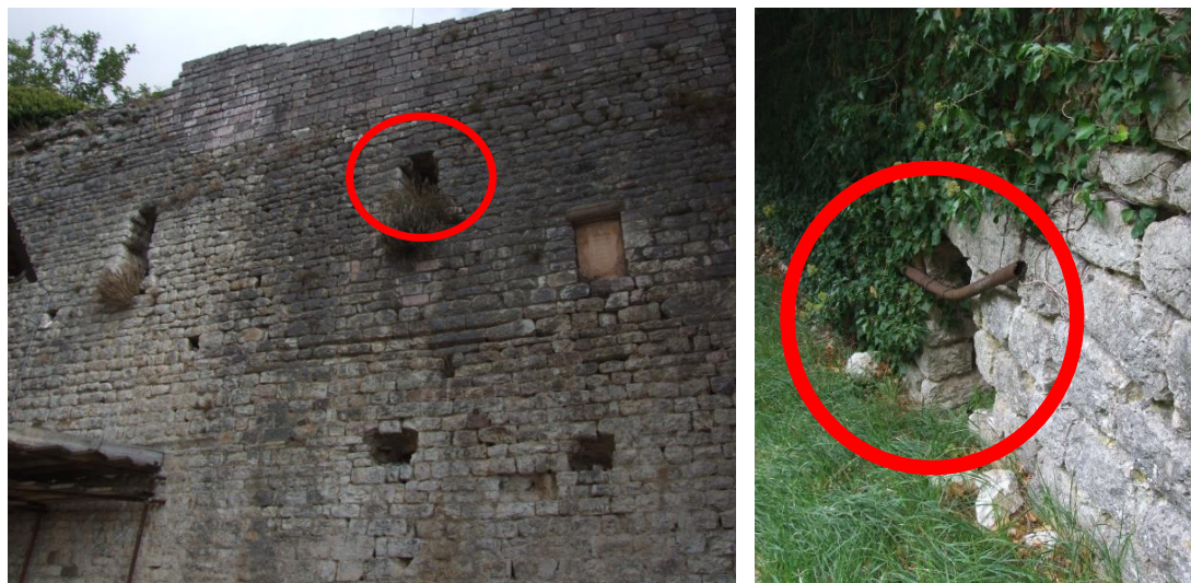
Figure 35: zone 4 (as in Fig. 15): Walls downstream side - notice the opening at around 6 metres from the ground level downstream.
