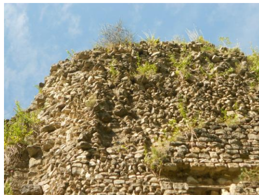
Figure 51 - erosion due to rainfall and degradation of mortars
