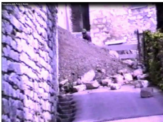
Figure 22 – 1985 collapsed terracing, with the landslide, in the zone 4 ("Porta S. Ubaldo"), view from below
