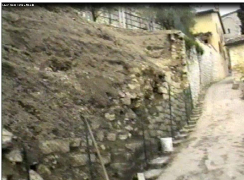
Figure 24 - 1985 collapsed terracing, after the removal of the collapsed material, view from below
