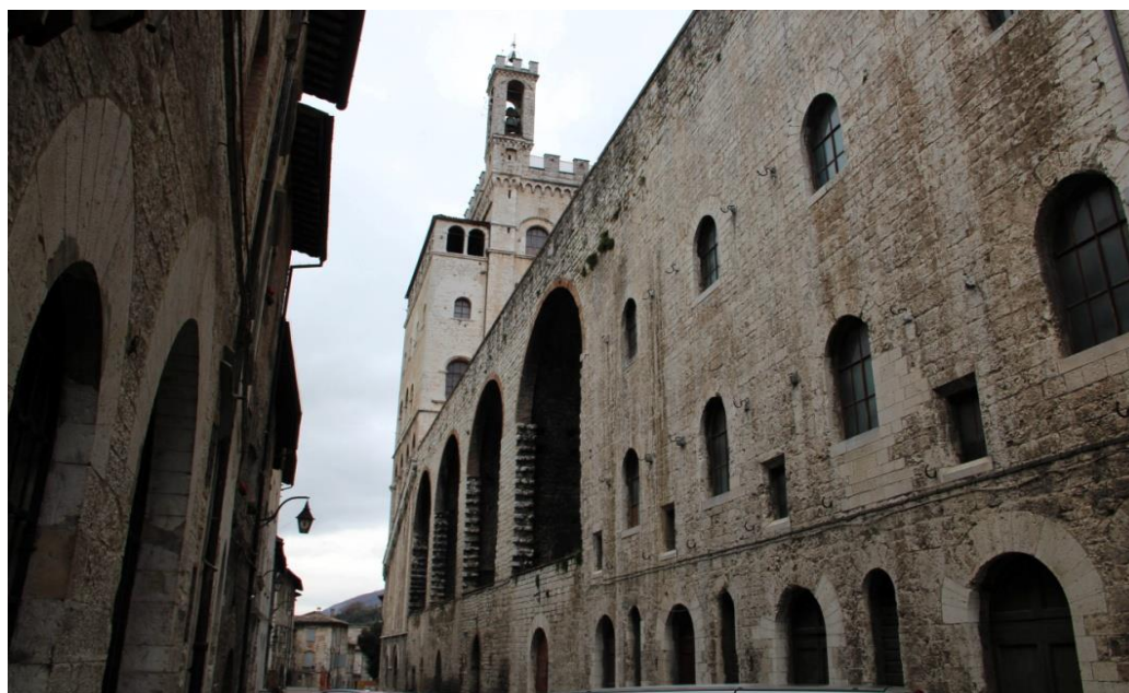
Figure 59 - Consoli Palace - black crusts on the façade, view from S-W side
