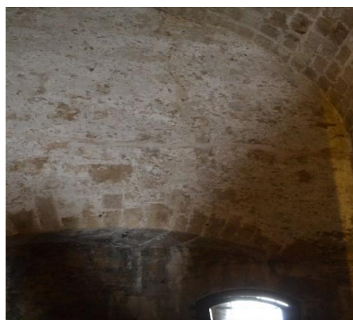
Figure 69: Crack at the room (26) next to “sperone”
