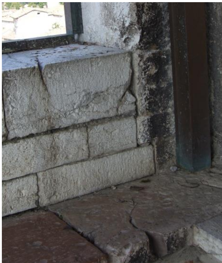
Figure 53 - cracks in loggia due to rocking mechanism
