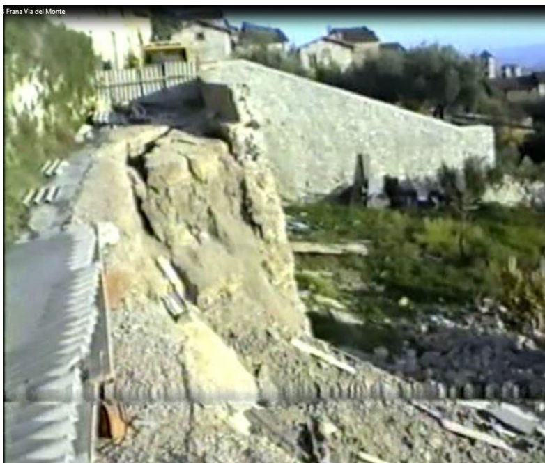
Figure 32 - collapse of the medieval terracing under the covering and extending for a greater area with respect to the former problem evidenced by the chasm – just below via del Monte (view from above- west side)
