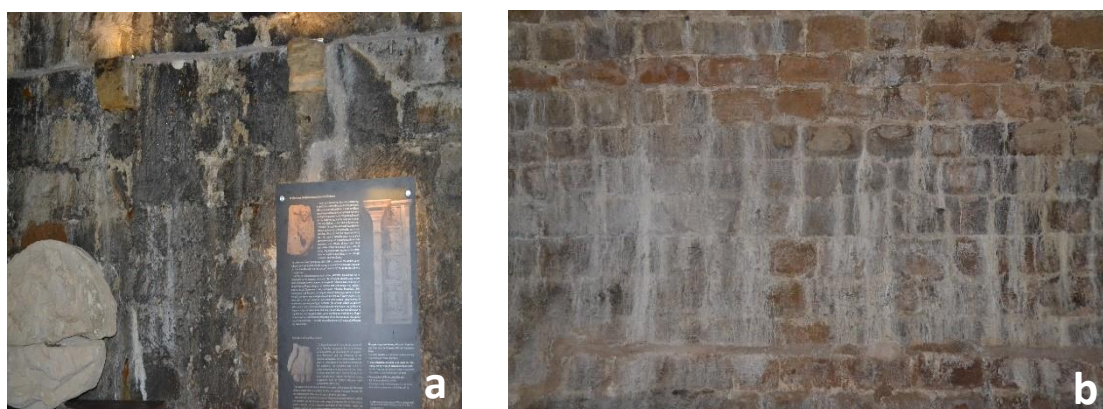
Figure 64 a) and b): Black crusts and salt efflorescence
