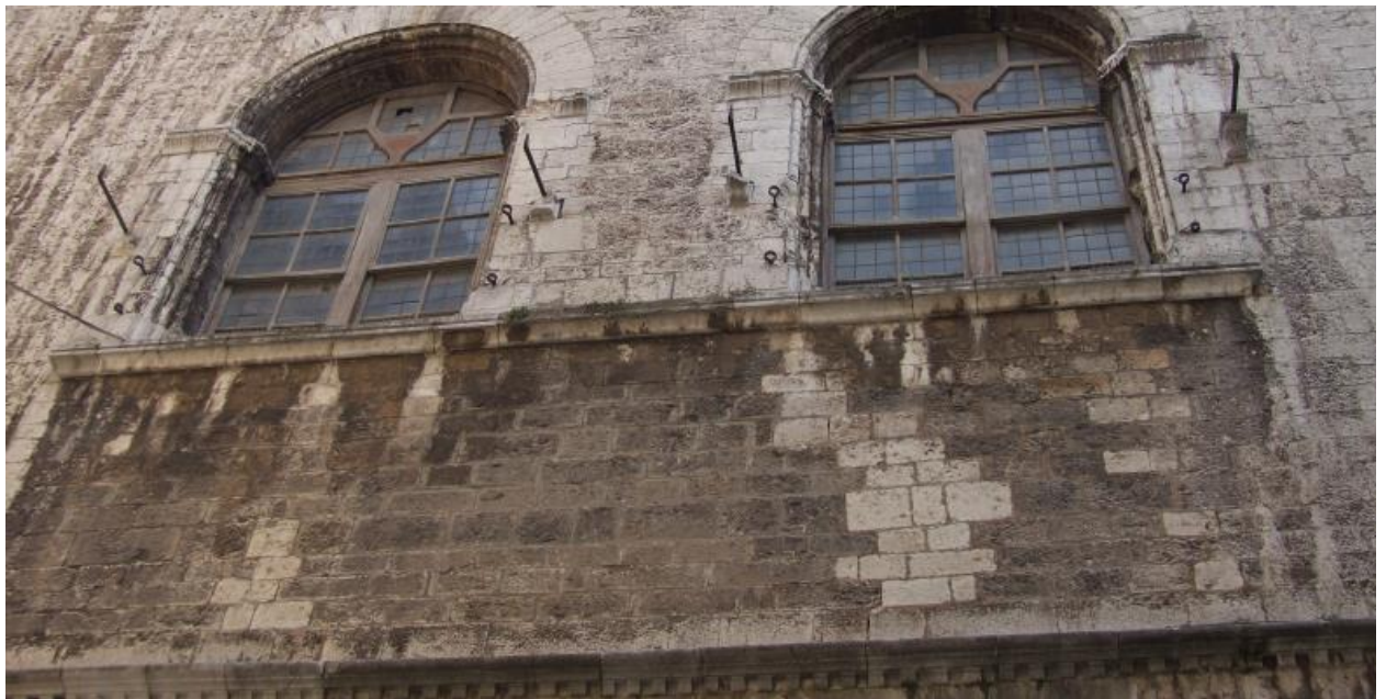
Figure 61 - Consoli Palace - black crusts on the façade, view from N-E side
