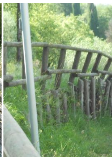
Figure 39- zone 3-4: ben bended/broken fence
