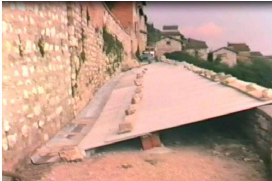
Figure 29 – covering of the chasm to prevent further possible negative effects induced by rainfall
