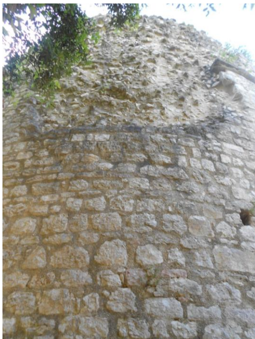
Figure 50- Zone 1 - tower restored before 1990: the mortars used are decaying and flaking and part of the external face collapsed
