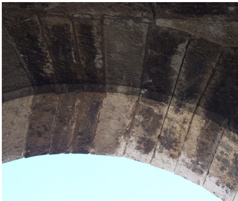
Figure 58 - Consoli Palace- arch of the loggia showing differential blackening (limestone)
