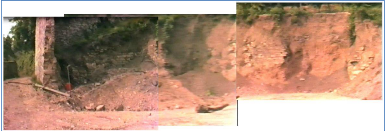
Figure 27 - Walls collapse upstream via del Monte
