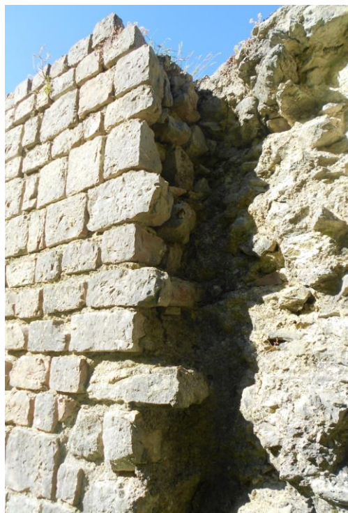
Figure 42 - zone 3 as indicated in Fig.15: - rainfall erosion
