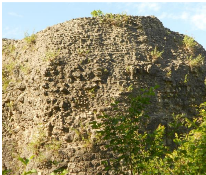
Figure 40 - zone 1 as indicated in Fig.15: effect of rainfall erosion on walls
