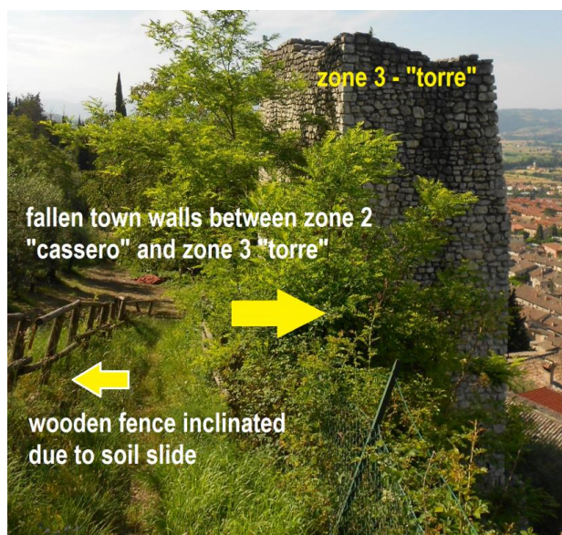
Figure 21: zone 3 (as referred to Fig.15) – zone were walls collapsed and bended fence due to soil pushing
