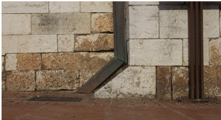
Figure 56 - blackening of materials (Piazza Grande level)
