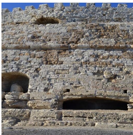
Figure 66: Crack outside the “sperone”
