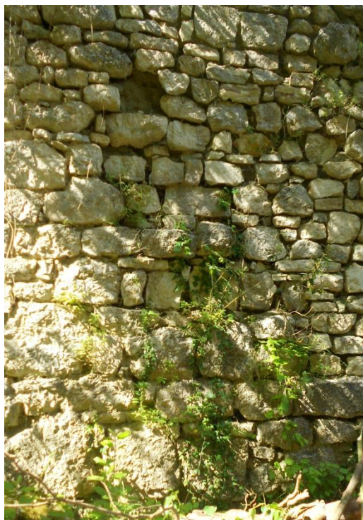
Figure 41 - zone 1 as indicated in Fig.15: - rainfall erosion
