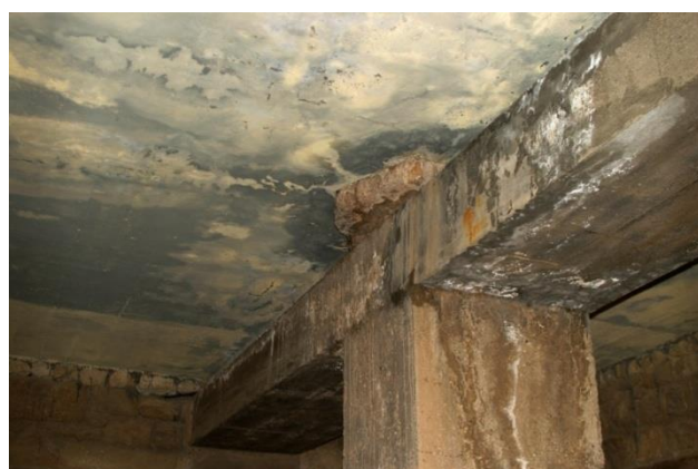
Figure 91. The results of the uncontrolled rain water drainage can be summarized as: erosion of the iron rebar, further degradation of the concrete building and ornamental elements, salt efflorescence, “Pillar Crypts”, Palace of Knossos
