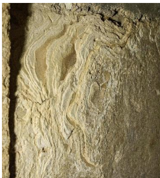
Figure 84: Delamination; Exfoliation of microcrystalline mineral gypsum slab, Knossos Palace
