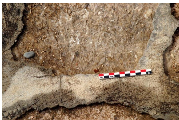
Figure 90. Rain water is channeled through the discontinuities to the substrate on which the gypsum elements are founded. The water flow contributes to further erosion and loss of material of the original parts of the monument, “King’s Megaron”, Palace of Knossos
