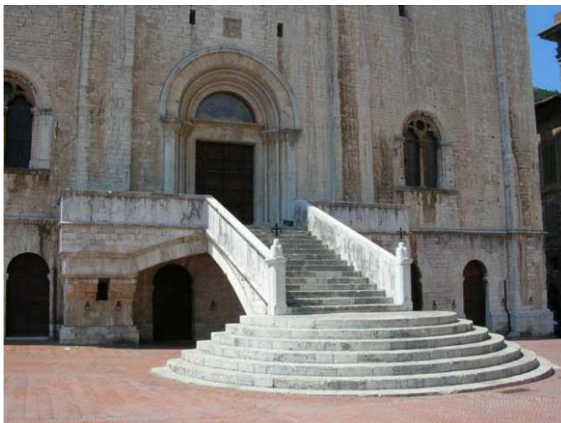
Figure 67: partial view of the Palace façade with the staircase, with evidences of the stones blackening
