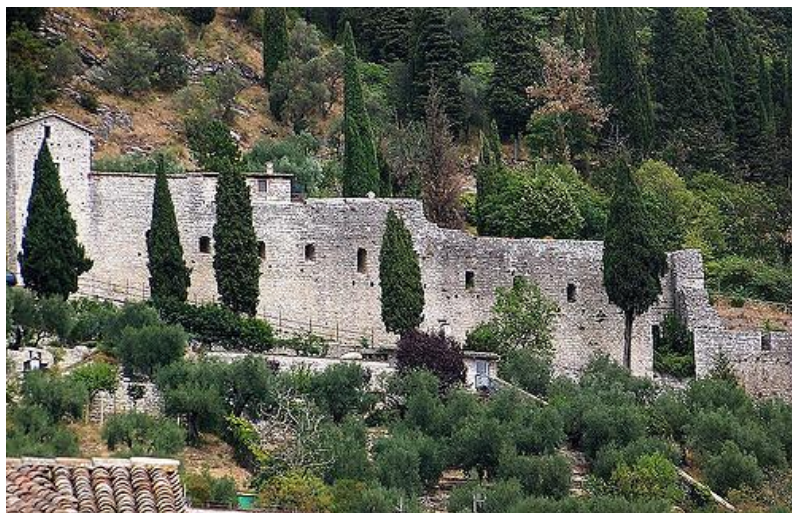
Figure 62: a partial view of the Gubbio Town Walls on the slopes of the Ingino mountain
