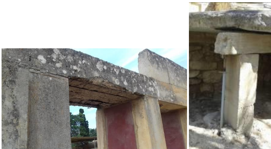
Figure 11: Corrosion of the iron reinforce used in Evans's reconstruction, degradation, deformation of reinforced concrete elements.
