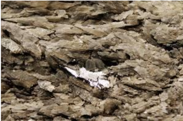
Figure 18: Loss of cohesion between gypsum (selenite) crystal aggregates leading to crumbling.
