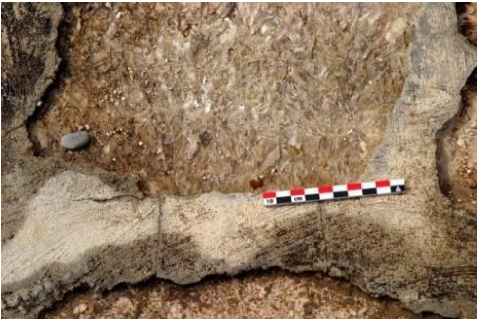
Figure 27: Rain water is channelled through the discontinuities to the substrate on which the gypsum elements are founded. The water flow contributes to the worsening of erosion effect and loss of material of the original parts of the monument, “King’s Megaron”, Palace of Knossos.
