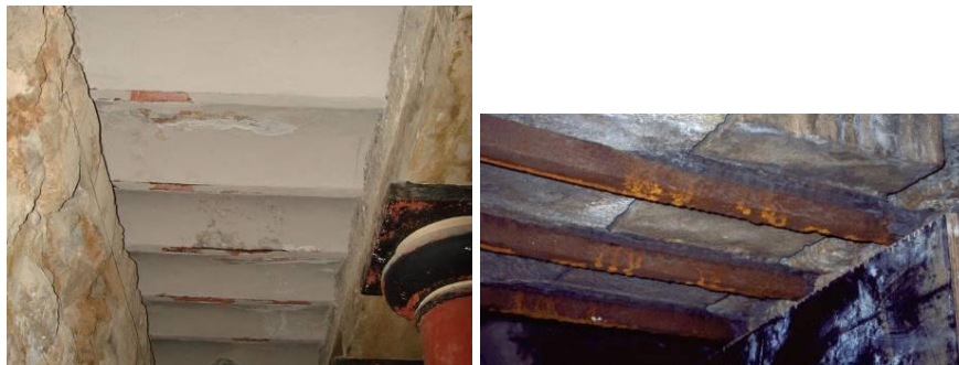
Figure 10: Corrosion of the iron girders used in Evans's reconstruction.
