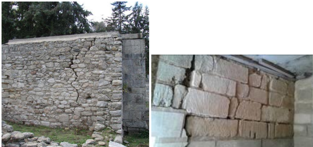
Figure 8: Cracking in restored and ancient wall.
