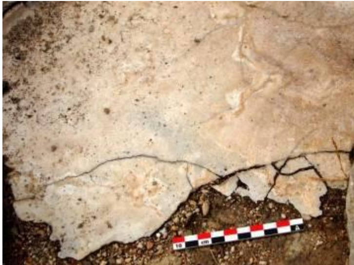
Figure 13: Secondary mineral gypsum from the Palace of Knossos showing a network of thin cracks.
