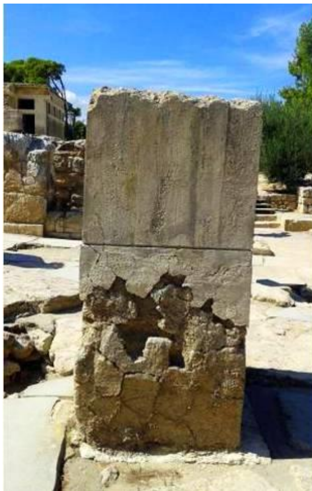
Figure 14: Fractures: Cracks due to mechanical stress. "North Entrance", Palace of Knossos.
