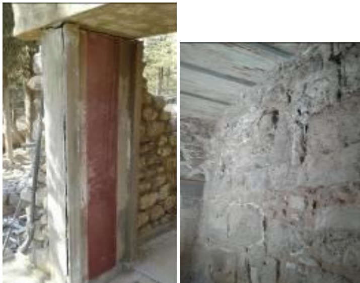
Figure 12: Deformation of reinforced concrete elements of Evans's reconstruction, efflorescence salts on the ancient and the restored masonry.
