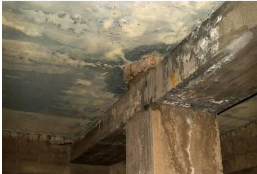
Figure 28: The results of the uncontrolled rain water drainage can be summarized as: erosion of the iron rebar, further degradation of the concrete building and ornamental elements, salt efflorescence, "Pillar Crypts", Palace of Knossos.
