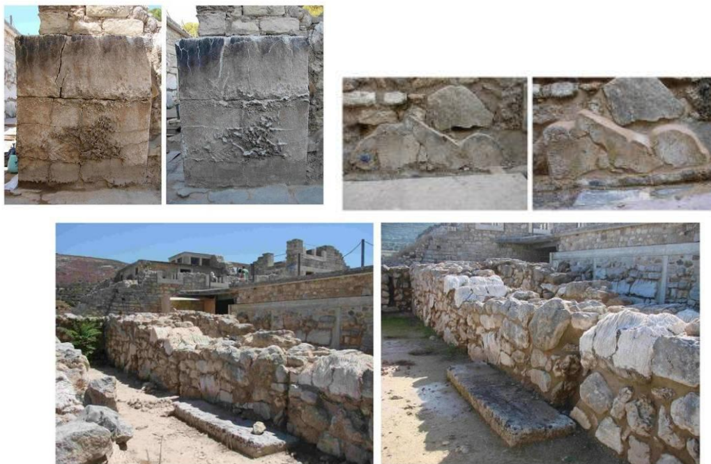
Figure 3: Palace of Knossos. Conservation of gypsum stones (selenite), ancient plaster of the Minoan masonry.
