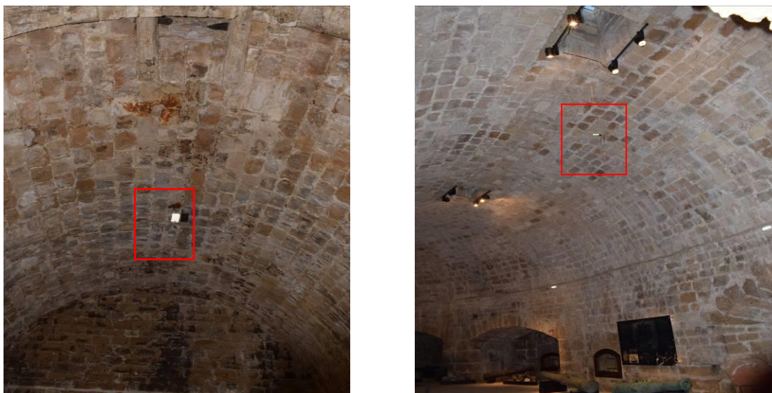
Figure 69: Data loggers for measuring RH and temperature, installed by FORT/IESL in rooms 11-12 and 24 (Sperone) at Koules fortress.
