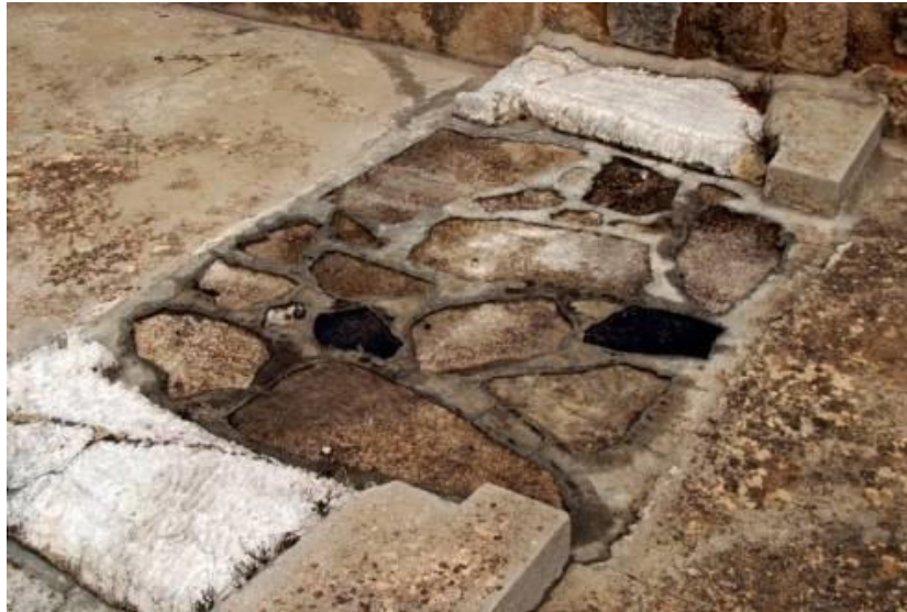
Figure 26: The dissolved gypsum elements are preserved in a lower level comparing to the cement mortar that was initially used for the fixation of the gypsum fragments, “King’s Megaron”, Palace of Knossos.
