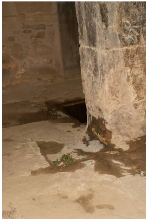
Figure 29: Salt efflorescence, of higher plantation growth and rain water accumulation, (after the rainfall on the 31st of October 2016), "Pillar Crypts", Palace of Knossos.
