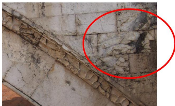
Figure 24 - Consoli Palace- main stairs - thermoclasts due to freeze-thaw/frost damage with loss of material (see red circle)
