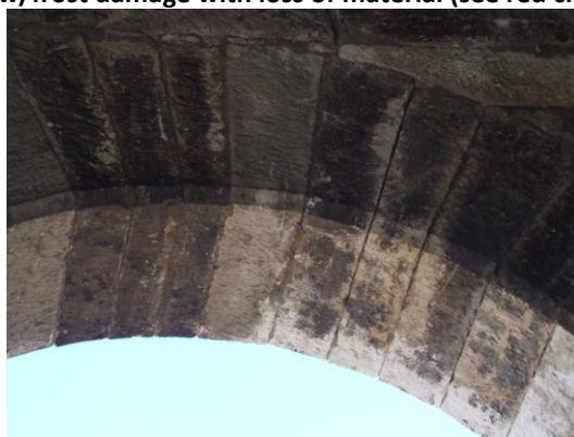
Figure 26 - Consoli Palace- differential blackening in the arch of the lodge
